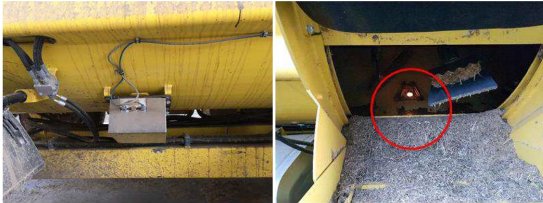
Fig. 1. NIR sensor mounted outside the mixing hopper (on the left); spectrometer measuring head at the bottom of the hopper and close to the unloading belt conveyor (on the right).
